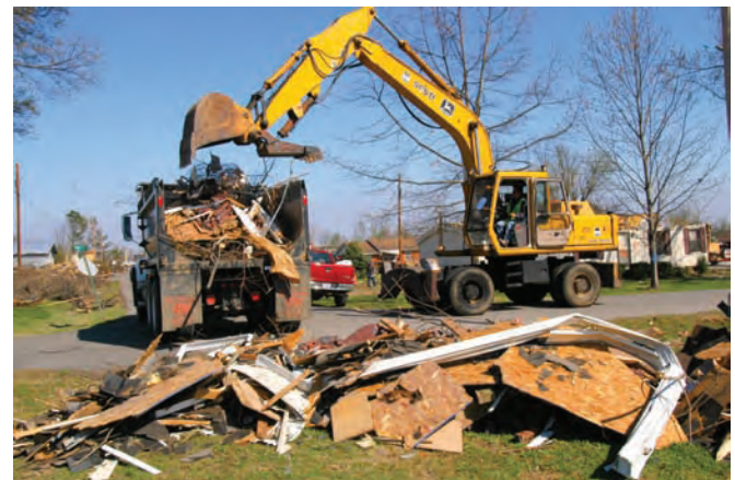
A back hoe clears debris in Marmaduke, Arkansas, after a tornado scattered debris everywhere. (FEMA photo by Win Henderson)
